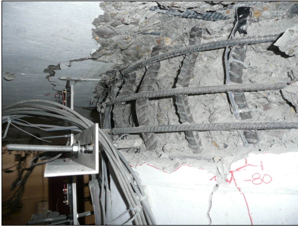
Figure 6.16: Buckling in the Top Column Hinge on the North Side at \mu_{\Delta}=10
