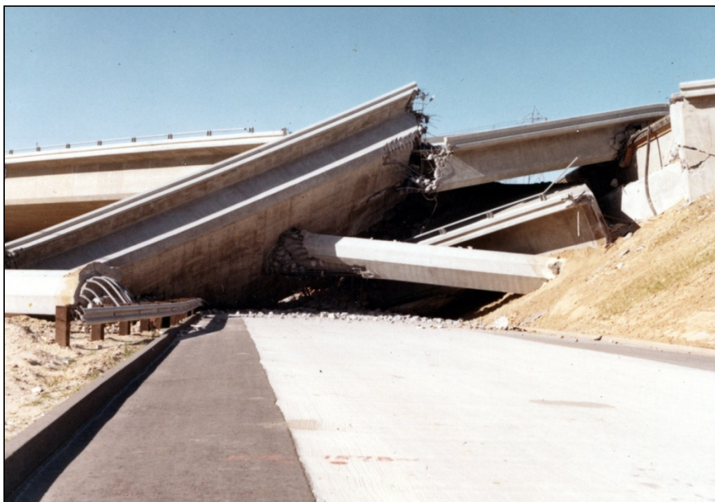
Figure 1.1: Example of 1971 San Fernando Earthquake Damage
