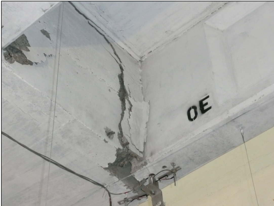
Figure 6.33: Damage to As-built Connection Exterior Girder at +2 in. Displacement
