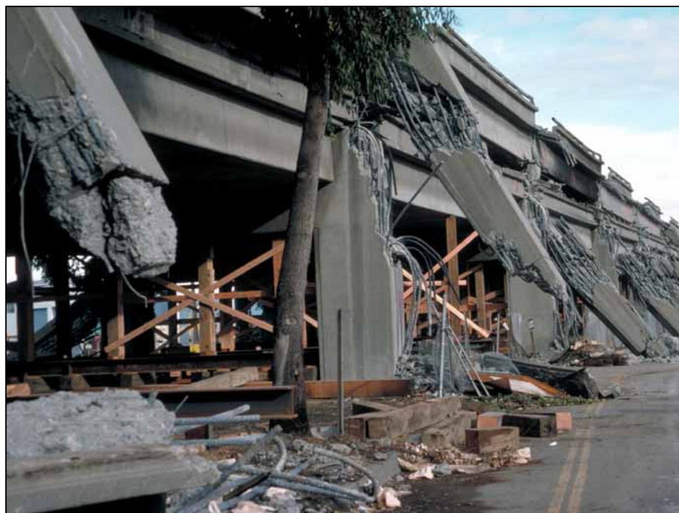
Figure 1.2: Example of 1989 Loma Prieta Earthquake Damage
